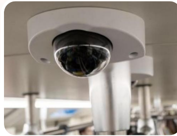
CCTV connected to OCC
